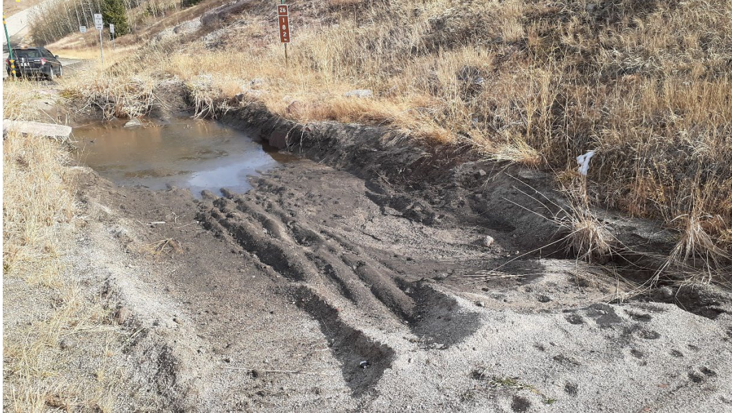
Figure 3.2 .Soft-sided Sediment Basin No. 26 on Westbound I-70
